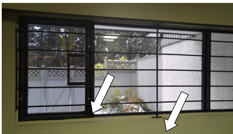
Asbestos containing black window mastic on the basement living room window and asbestos containing drywall in Unit 3033
