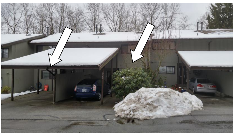
Lead containing green/blue and brown paint on the exterior of a Unit on Clarina Place
