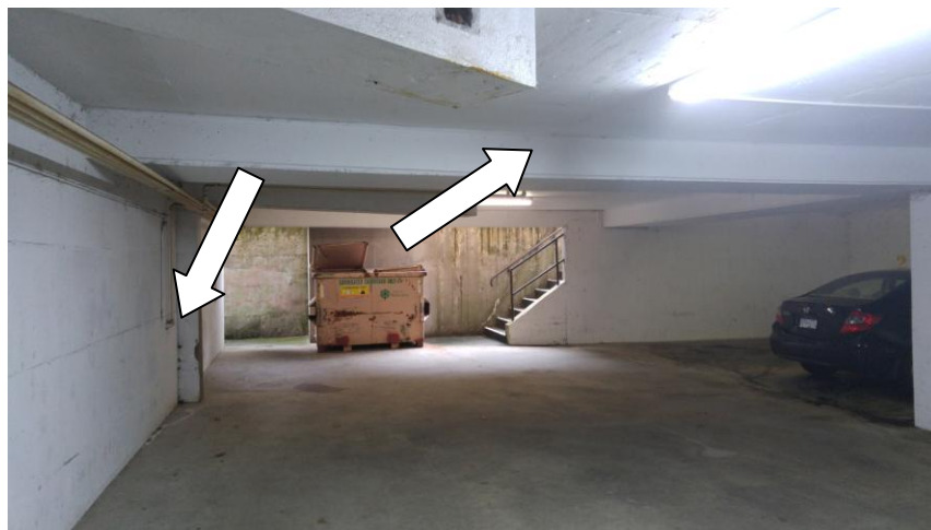
Non-asbestos containing stucco and lead containing white paint in the parkade
