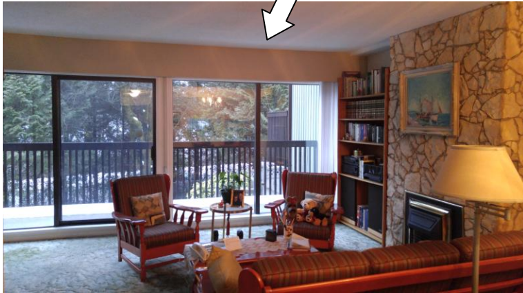
Asbestos containing ceiling texture and drywall in the main floor living room of Unit 3033
