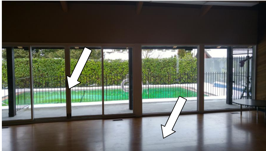
Asbestos containing window glazing mastic on the pool house exterior windows and asbestos containing vinyl flooring in the pool house main area/kitchen
