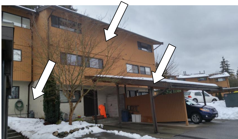
Lead containing orange and brown paint with non-asbestos containing stucco on the exterior of a unit on Clarina Place
