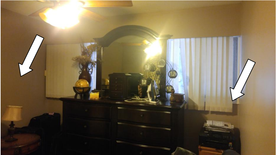
Asbestos containing black window mastic on the 3 rd floor bedroom window and asbestos containing drywall in Unit 3036
