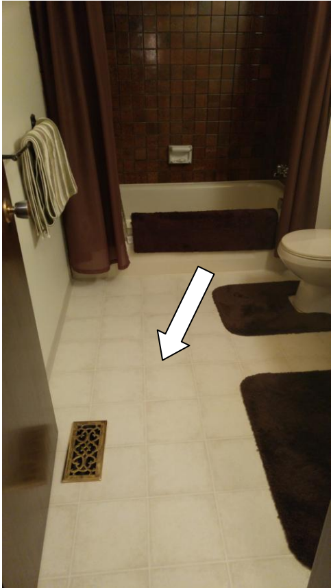
Asbestos containing Linoleum sheet flooring in the upper floor bathroom of Unit 3033
