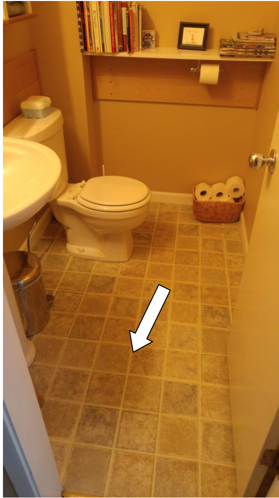
Asbestos containing Linoleum sheet flooring in the upper floor bathroom of Unit 3032
